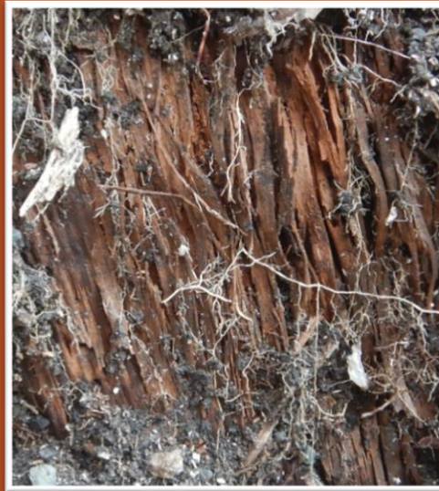
Wood plank drying and cracking
